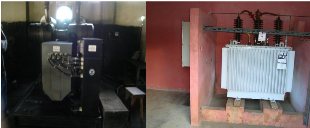
(Genset and Transformer in Inhambane Mozambique)
