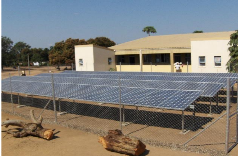
PV systems in Muxúngue Rural Clinic in Sofala, Mozambique
